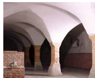
The interior walls of these buildings were restored with KÖSTER Restoration Plaster White.
