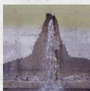
For water bearing cracks
