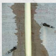
Forms foam in wet cracks
