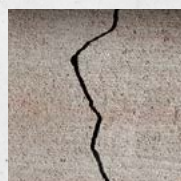
For dry cracks
