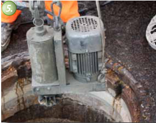
5. The material is mixed inside a mortar pump and then pumped into a special application tool. This tool is a rotating spiral, which literally shoots the material onto the...
