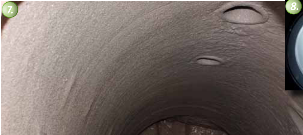
7. The ready coated shaft. A comparably smooth and homogeneous surface is achieved.
