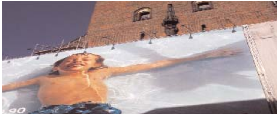
Fig. 1: city centre of Hamburg – H & M billboard as protective cover for work scaffolding
