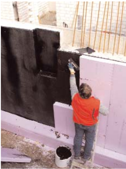
Fig. 4: When waterproofing a basement from the outside, the following details have to be observed: execution of the base area with rot-proof insulation. The transition from the masonry to the foundation is executed as a rounded out fillet. Important: the fillet must have dried prior to application of the primer. The thick film sealant can delaminate if it is applied on a fresh fillet which then shrinks during its drying process. The planning folder of the company DÖRKEN on the DELTA-system contains very good detail solutions and drawings.
